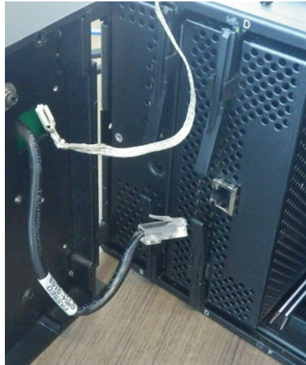
Figure 10-16: Disconnected ground cable and CPU connector
